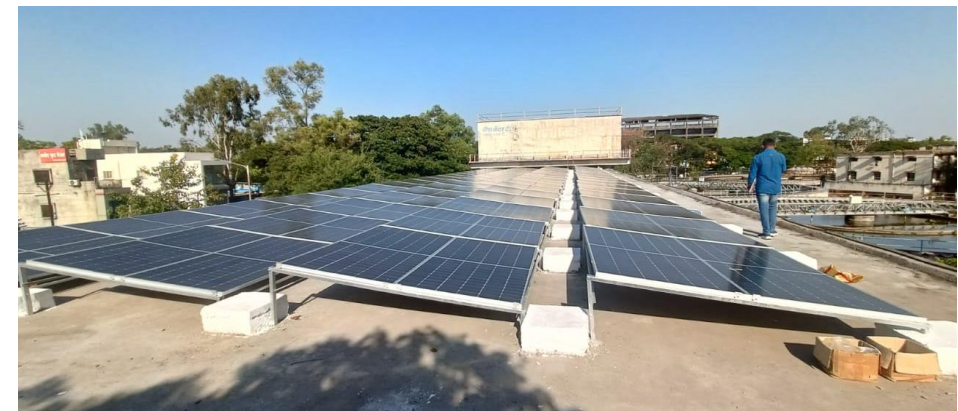
Ichalkaranji : 81 Kw at WTP
