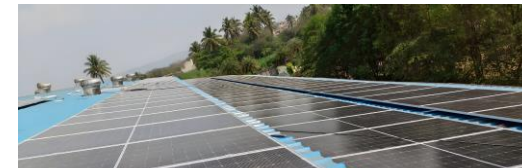
Karad : 72 Kw at STP
